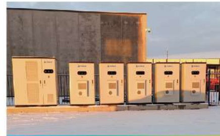
Equipment Rental Company, Norway Capacity: 500kW / 1075kWh Application: Peak Shaving, Balancing Services
