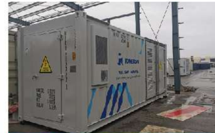
Electrical Equipment Factory, Mexico Capacity: 187.5kW / 648kWh Application: Solar Self-consumption
