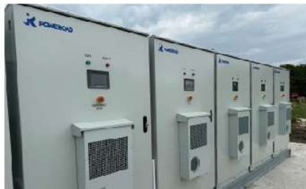
Pig Farm, Netherlands Capacity: 1.5MW / 3MWh Application: Balancing Services
