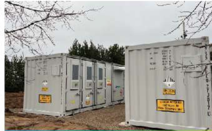
PV Panel Factory, Lithuania Capacity: 1000kW / 2580kWh Application: Solar self-consumption, Peak Shaving
