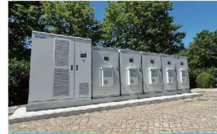
Glass Factory, Netherlands Capacity: 500kW / 1000kWh Application: Solar Self-consumption
