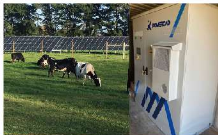
Dairy Farm, New Zealand Capacity: 60kW / 122.88kWh Application: Off-grid, Solar Self-consumption
