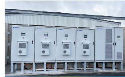
Steel Processing Factory, Sweden Capacity: 500kW / 860kWh Application: Frequency Regulation
