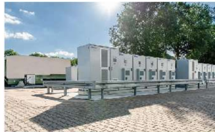
Logistic Fleet Charging Station, Netherlands Capacity: 1.5MW / 3.2MWh Application: Solar Self-consumption, Balancing Services
