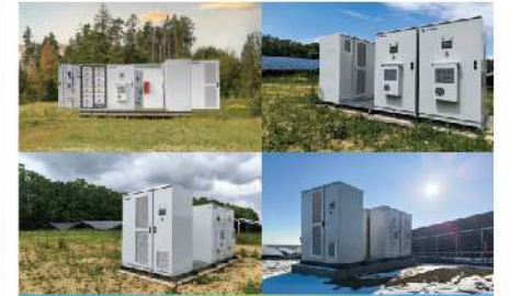
PV Power Station, Czech Capacity: 7MW / 12.47MWh Application: Solar Self-consumption
