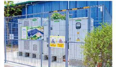
Engine Lubricant Factory, Vietnam Capacity: 100kW / 215kWh Application: Solar Self-consumption
