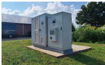
Livestock Farm, Netherlands Capacity: 62.5kW / 215kWh Application: Solar self-consumption, Balancing Service
