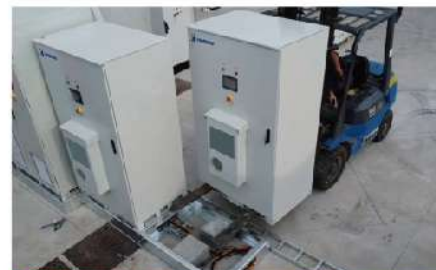
Chicken Farm, Belgium Capacity: 250kW / 430kWh Application: Balancing Services
