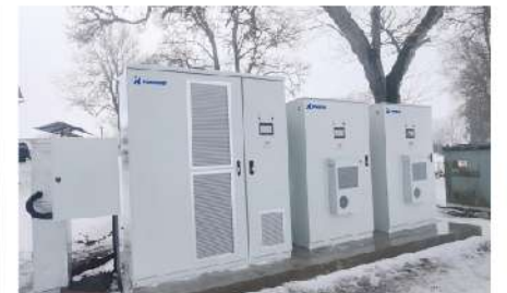
Sweden Capacity: 187.5kW / 430kWh Application: Frequency Regulation
