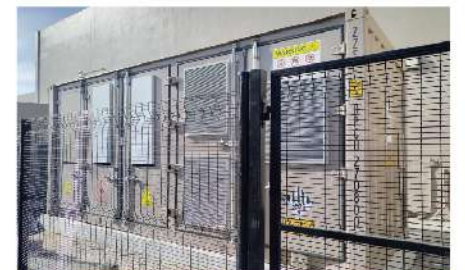
Shopping Mall, South Africa Capacity: 375kW / 860kWh Application: Backup Power
