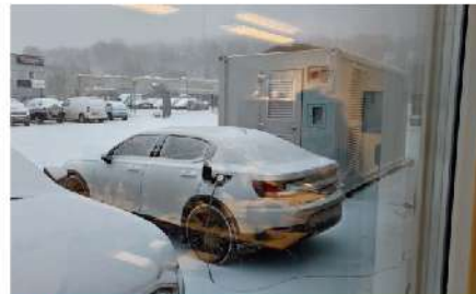
EV Charging Station, Sweden Capacity: 500kW / 504kWh Application: Demand Response
