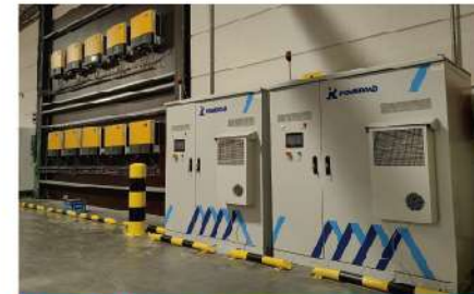
Chocolate Factory, Belgium Capacity: 350kW / 748kWh Application: Backup Power
