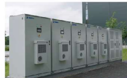
Distribution Center, Germany Capacity: 500kW / 1000kWh Application: Solar Self-consumption
